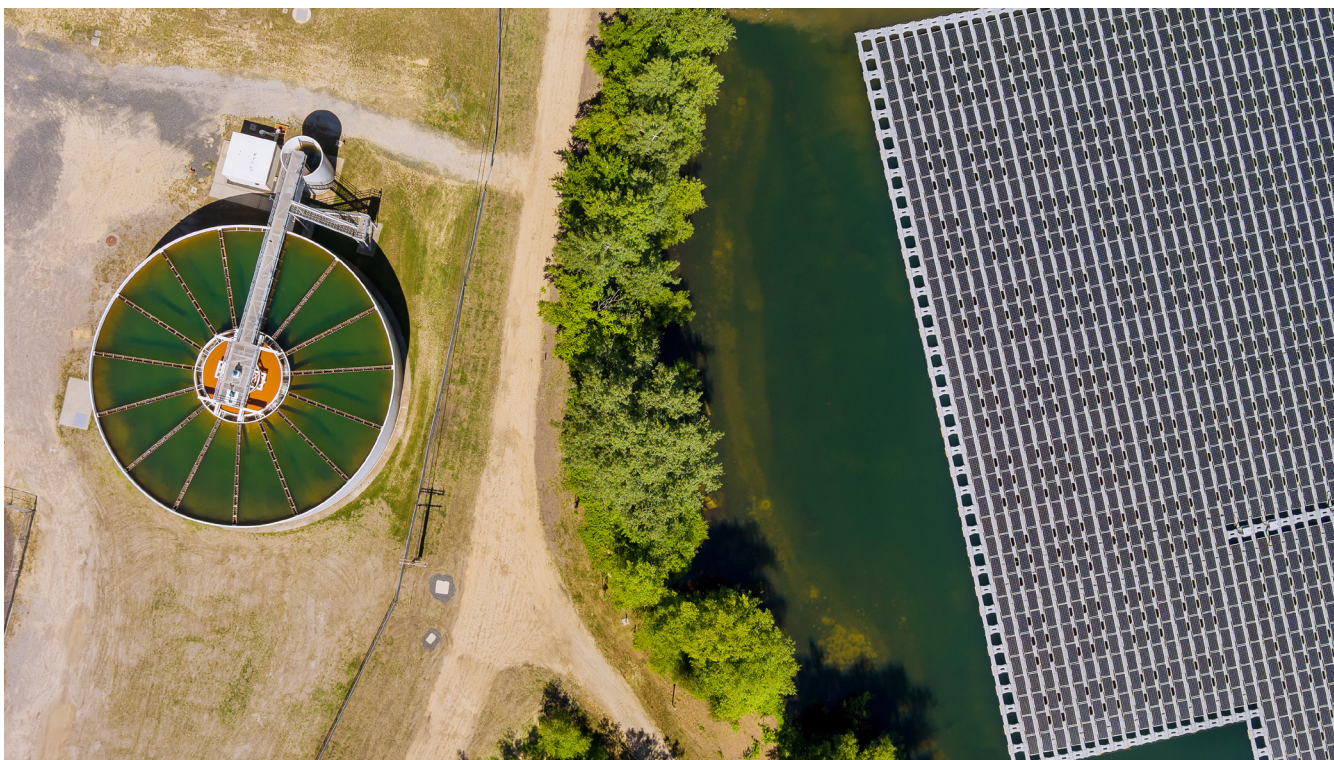
Decentralised wastewater treatment tank and floating solar farm. Source: Shutterstock.
